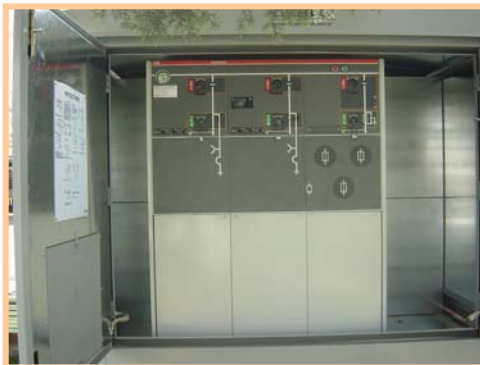
MV Switchgear Department
